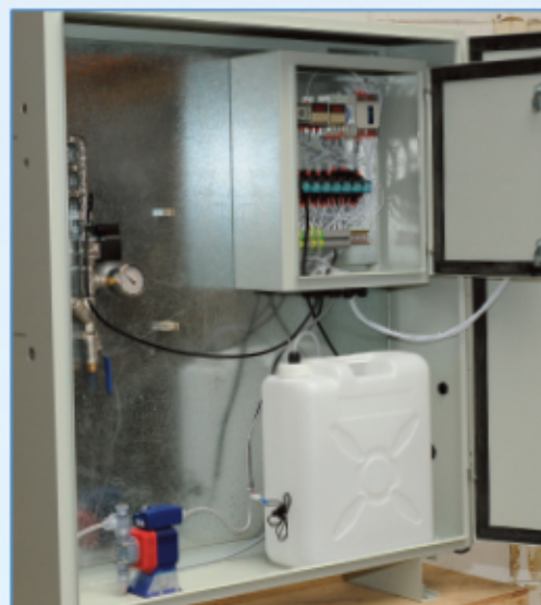
INTERIOR OF AUTOWASH CABINET
